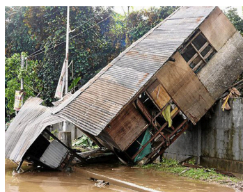
A house rests on a wall by the roadside in Cagayan de Oro City, a mute witness to the power and fury unleashed by Tropical Storm "Sendong." CAI PANLILIO/Inquirer Mindanao
